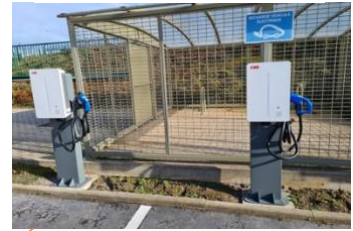
EDF offices of Maxéville Near Nancy, France
