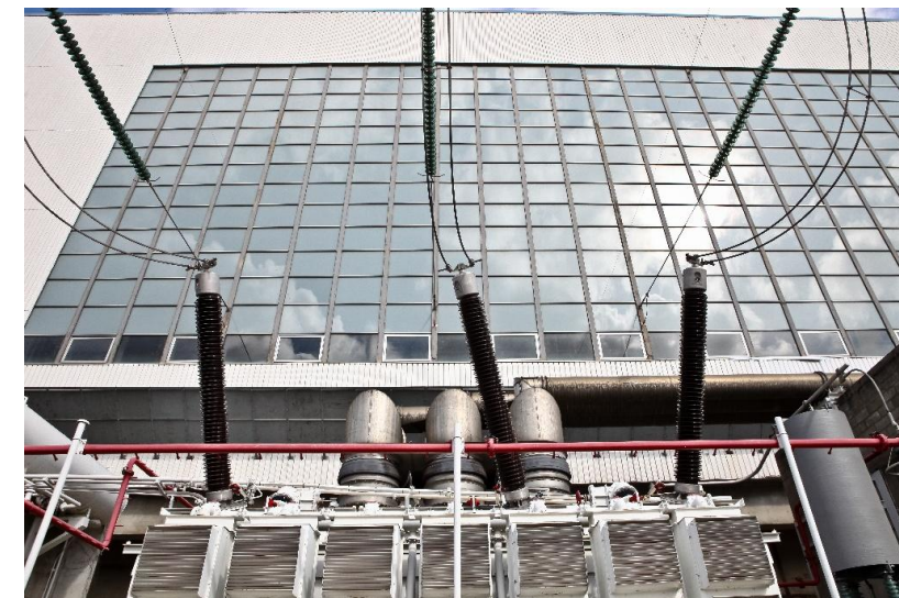
Porcheville electrical substation
