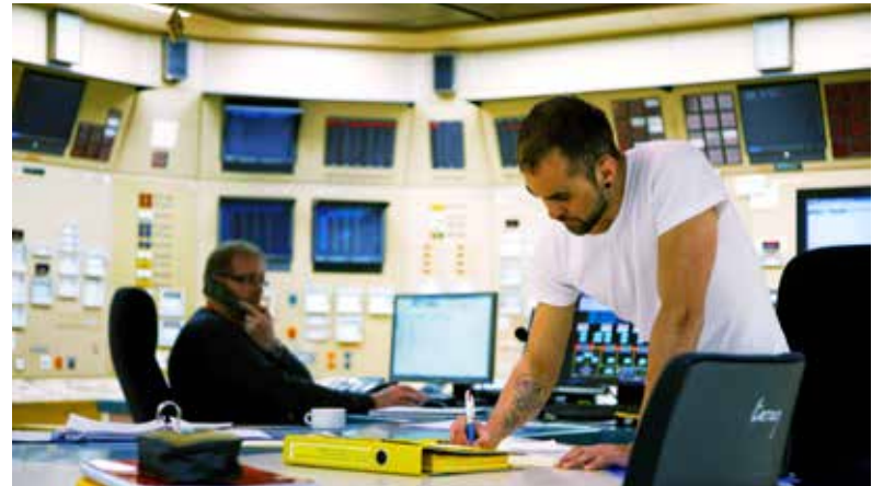
Control room operators - Flamanville nuclear power plant
