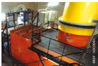
Incinerator in CentraCo.
