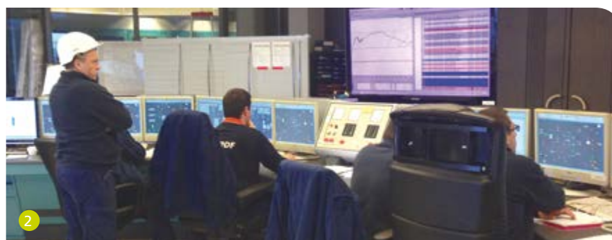
2 The control room in the Seraing plant. This combined cycle is a "black-start" production unit, which can start up without any external electricity source, thanks to its diesel generators. These generators are regularly started up in order to test them.
